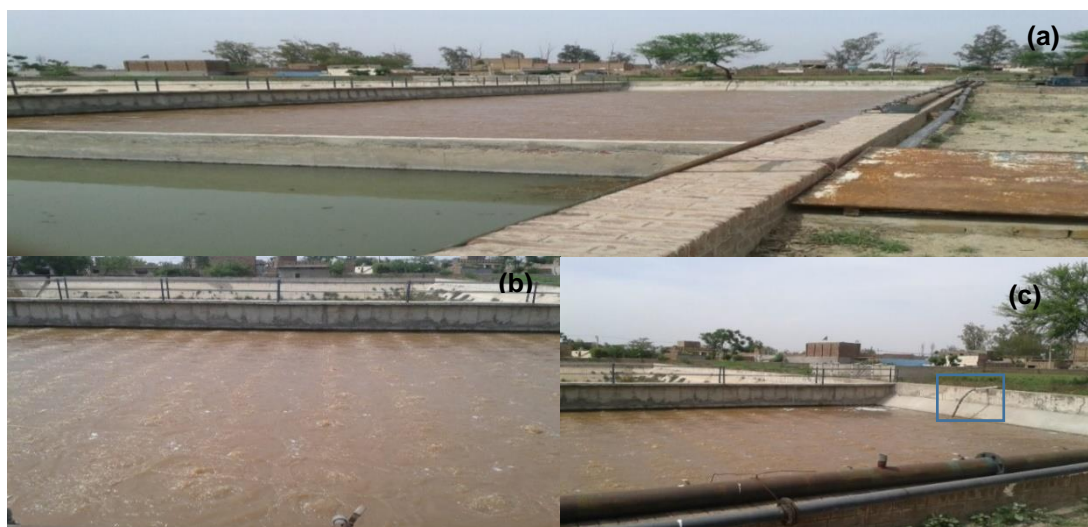
Figure 3.2 (a) Effluent treatment plant at Verka milk plant, Bathinda. (a) Aeration tank (b) close view of aeration tank (c) Return sludge.
