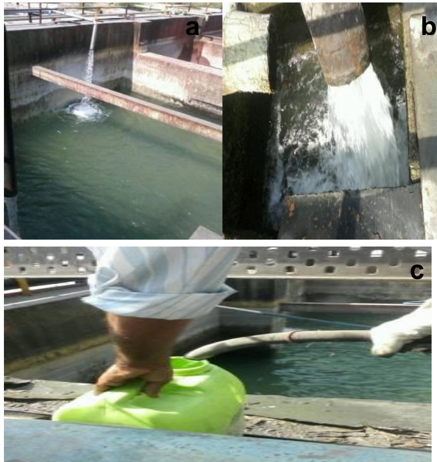
Figure 4.1 (a) Wastewater flowing out of pipelines, (b) Close view and (c) Wastewater Collection
